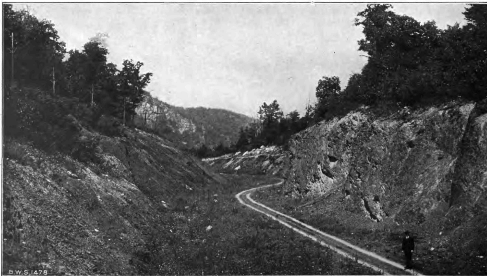
CATSKILL AQUEDUCT—Wallkill North cut-and-cover aqueduct, looking north toward South portal of Bonticou tunnel; completed backfilling over aqueduct in Freer cut
