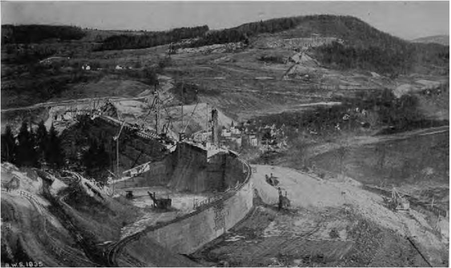
1924. Gilboa dam and dike, looking eastward from the end of the dike. Three steam shovels were used to handle the material dumped from the core-wall or trestle into wagons for evenly spreading the fill. Imagine sitting in those buildings and looking up at the dam! Photograph scanned from the Annual Report of the Board of Water Supply for 1924 , used courtesy of Department of Environmental Protection.
