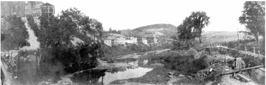
A 1919 panoramic view of the Gilboa valley looking south from the creamery site. The diversion of Steen Kill creek is on the right, and the initial stages of the mixing plant construction is on the top left of this picture.
